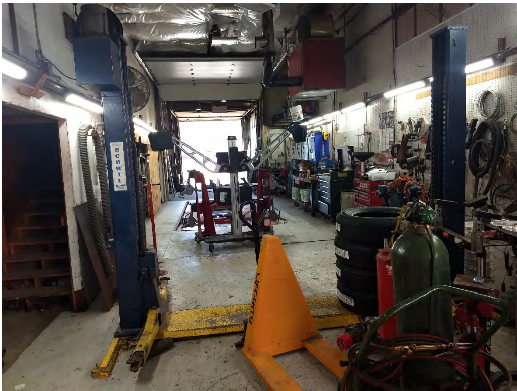
Additional aboveground vehicle lift.
