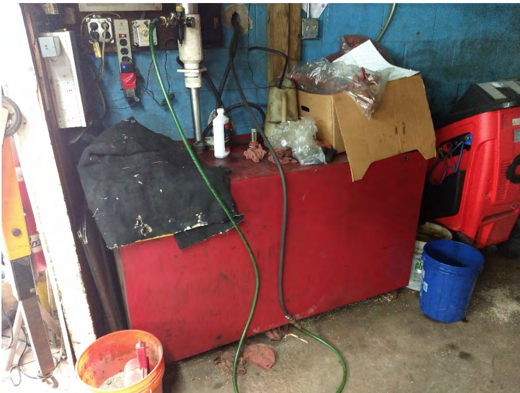
Waste oil storage tank in central portion of 118 Broadway garage.
