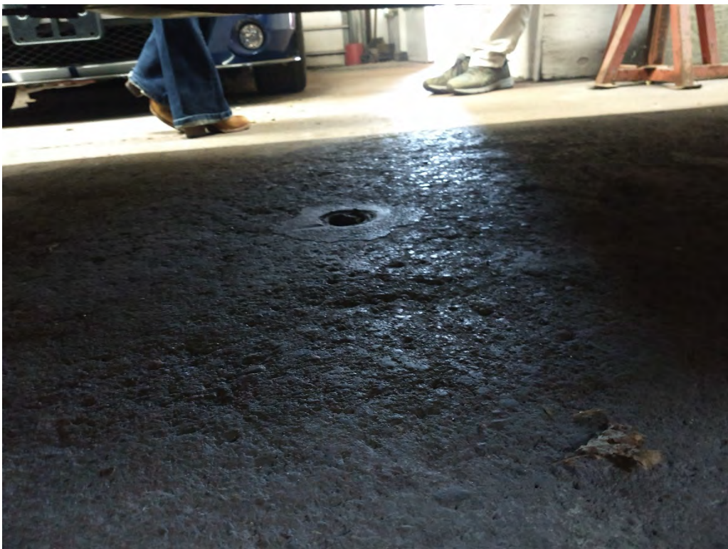
Sealed floor drain under vehicle at 116 Broadway.
