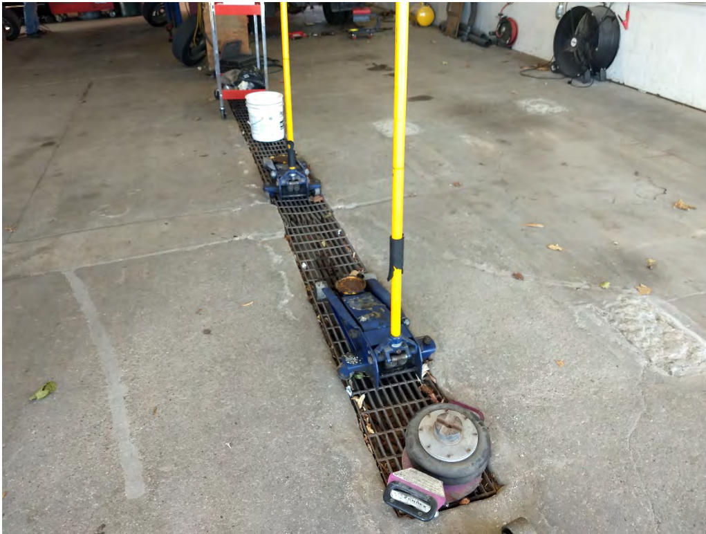
Trench drain in south service bay at 118 Broadway.
