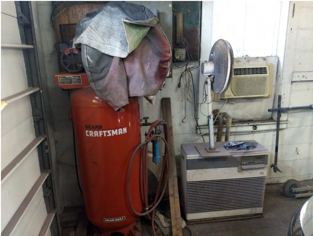
Air compressor and space heater inside garage at 116 Broadway.
