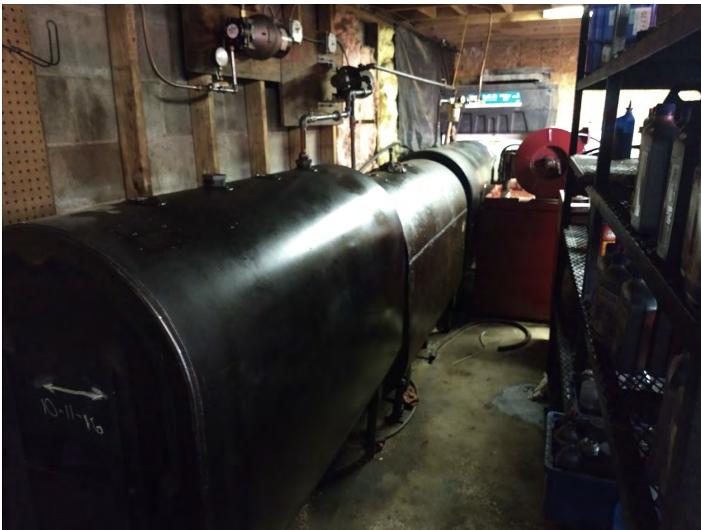
Three (3) 275-gallon waste oil ASTs and additional 300-gallon waste oil AST.
