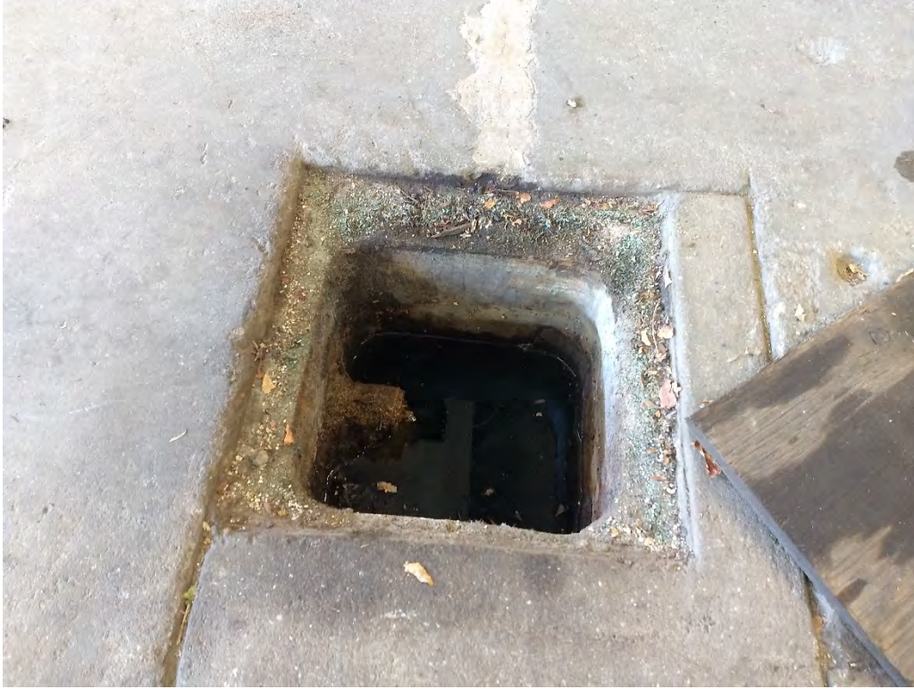
Floor drain with cover removed and water in bottom.
