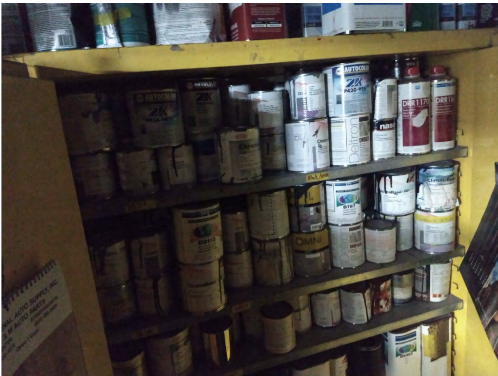
Containers inside flammable storage cabinet at 116 Broadway.
