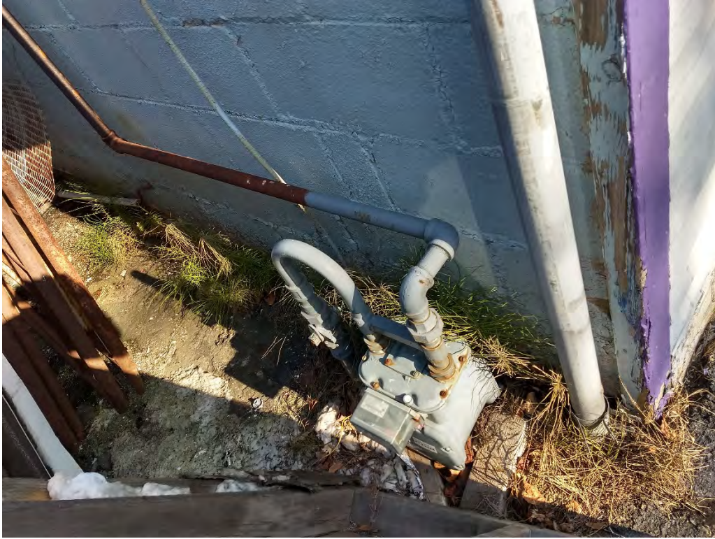
Natural gas meter on north side of #116 Broadway.
