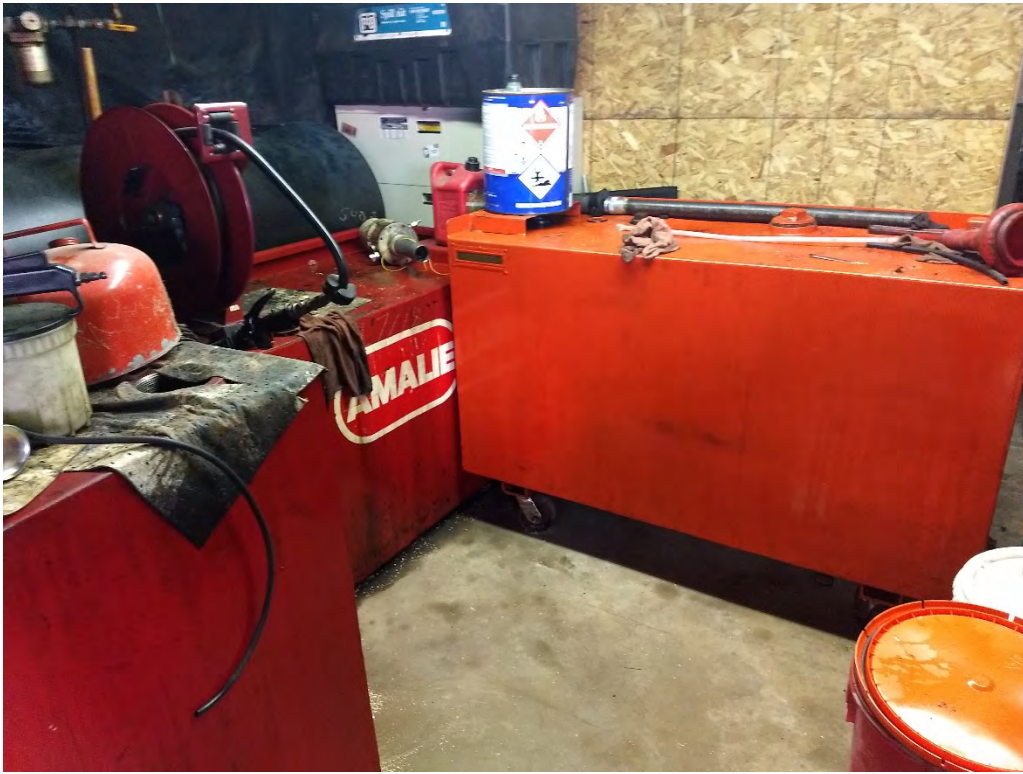
Three (3) waste oil storage tanks with minor staining on floor.
