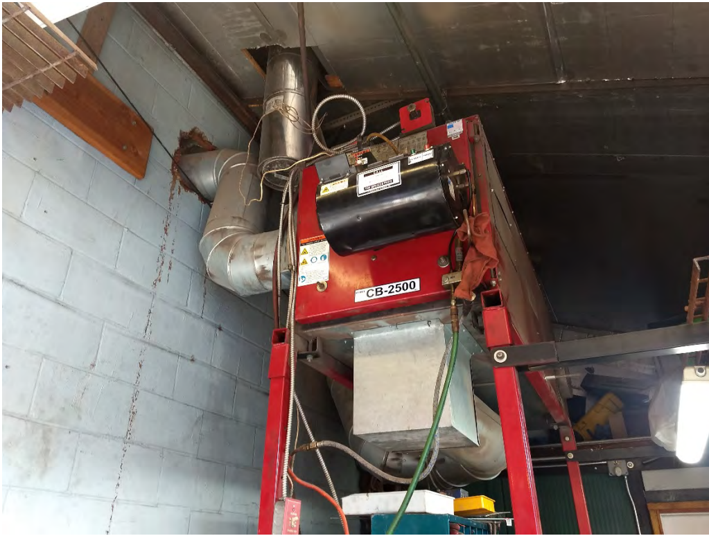
Waste oil furnace in central portion of 118 Broadway building.
