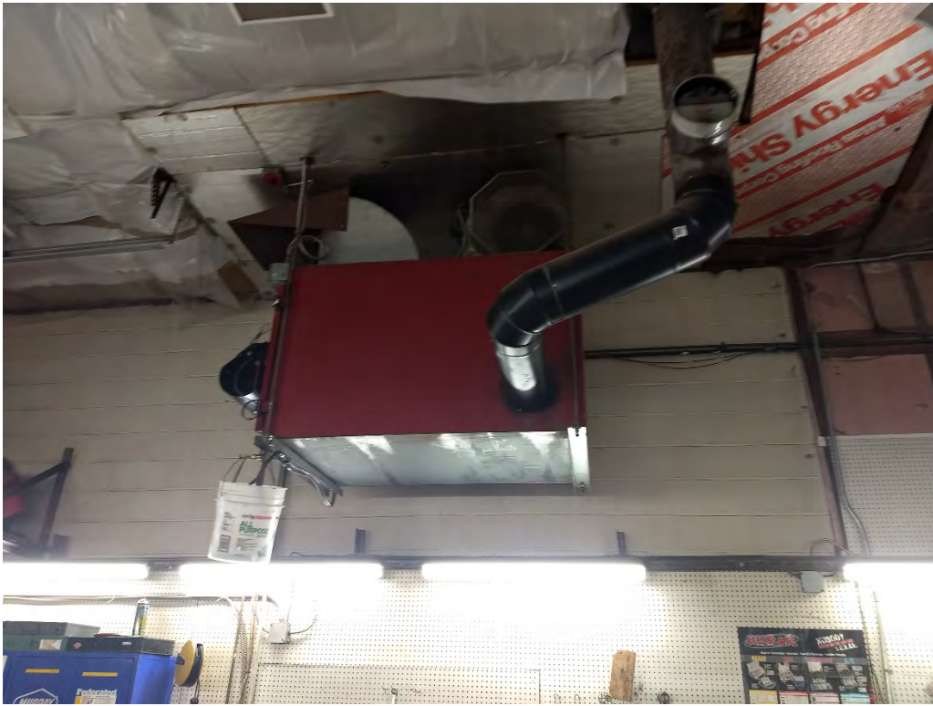
Additional overhead waste oil furnace.
