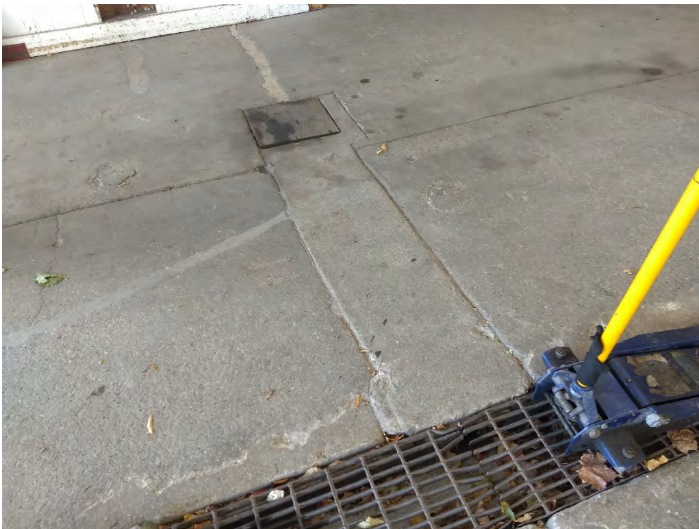
Trench drain with adjacent floor drain.
