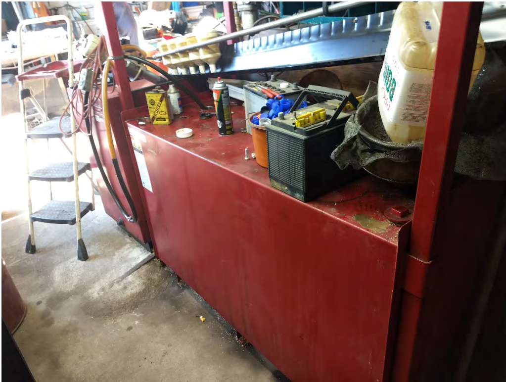
Two (2) waste oil tanks in central portion of 118 Broadway garage.
