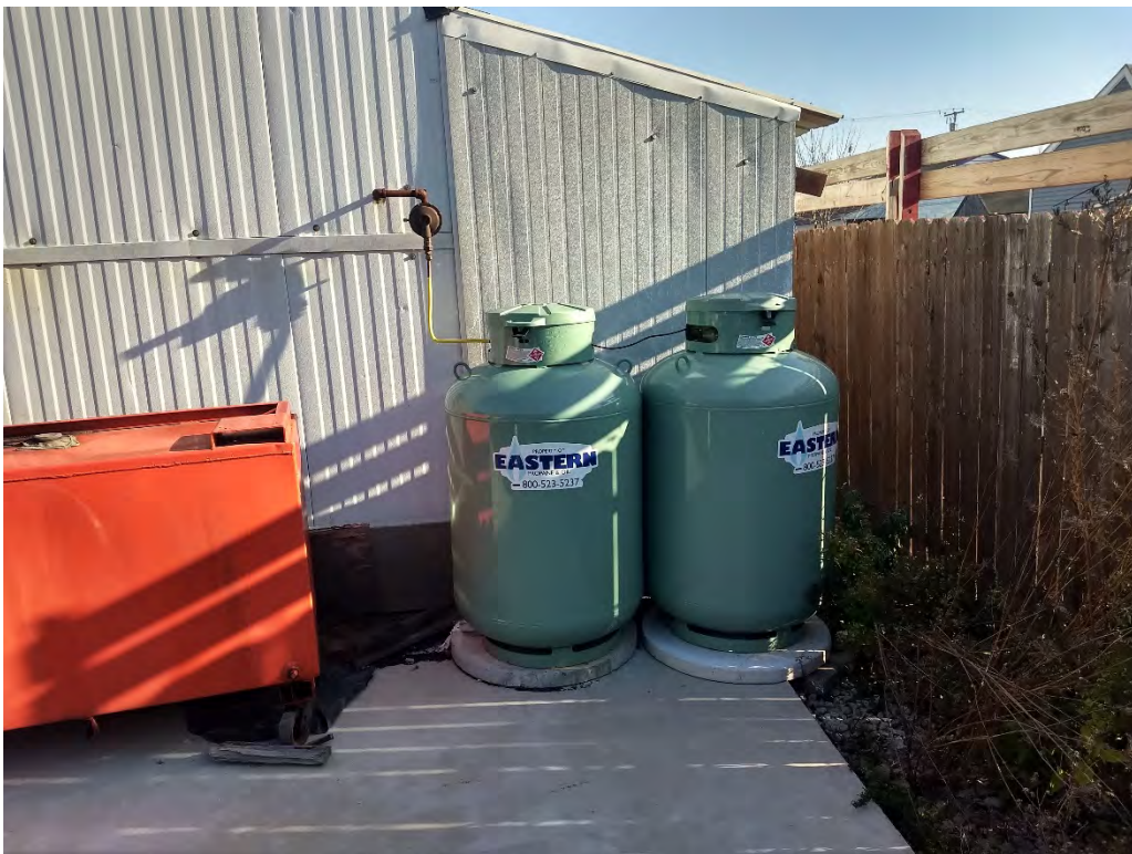
Propane tanks on north side of 118 Broadway building.
