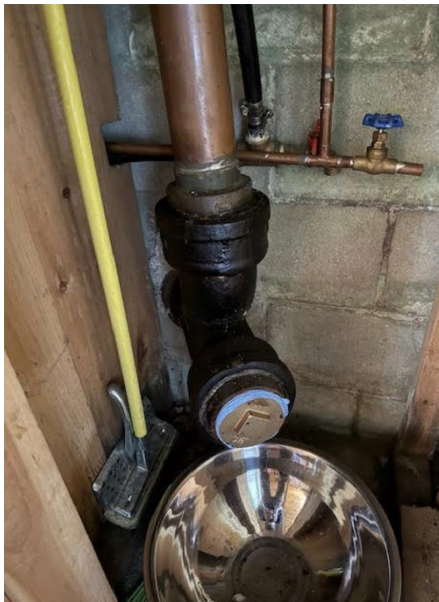
Interior Plumbing - Main Cleanout
